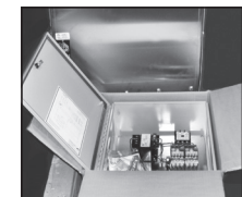
Inside the Control Panel enclosure (if supplied).
